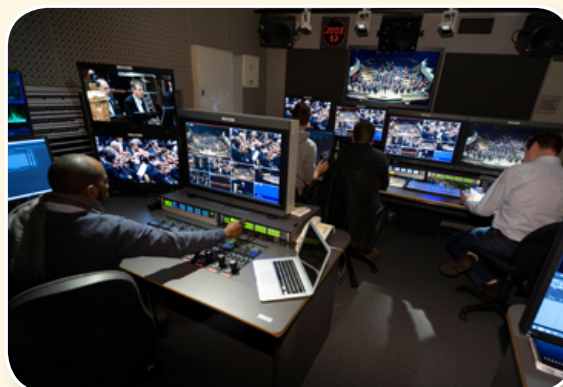
The Digital Concert Hall control room.
